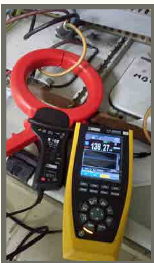
Measurement with leakage current clamp and recording of the fault.
