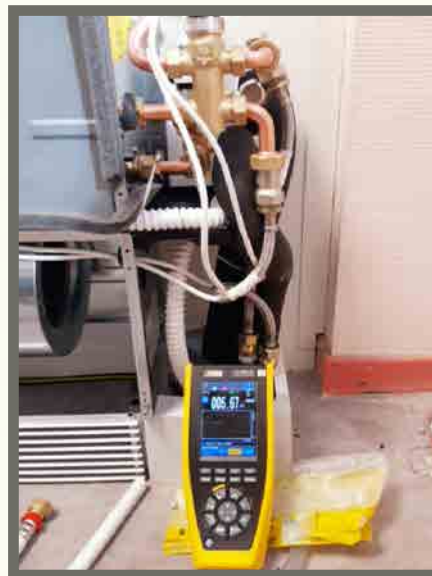
Measurements on heating and air-conditioning systems: current, voltage and temperature.
